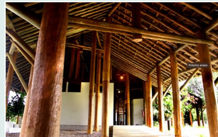
Images of the Center for Environmental Protection in Balbina (AM), now in ruins.
